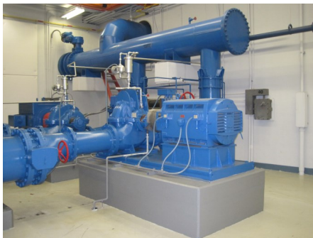
New City Distribution Pump at Water Treatment Plant
