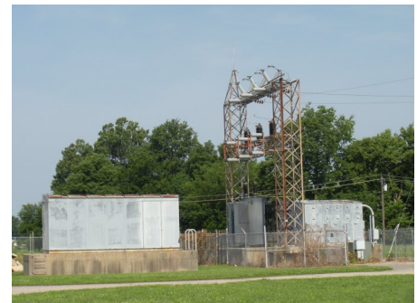
Aging High Voltage Subgear
