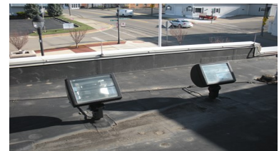
New Outdoor Building Lighting
