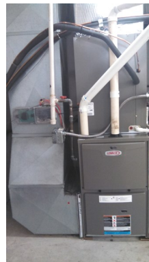
New Mechanical Systems
