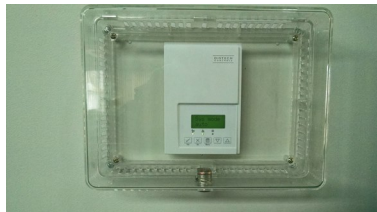
New Direct Digital Controls
